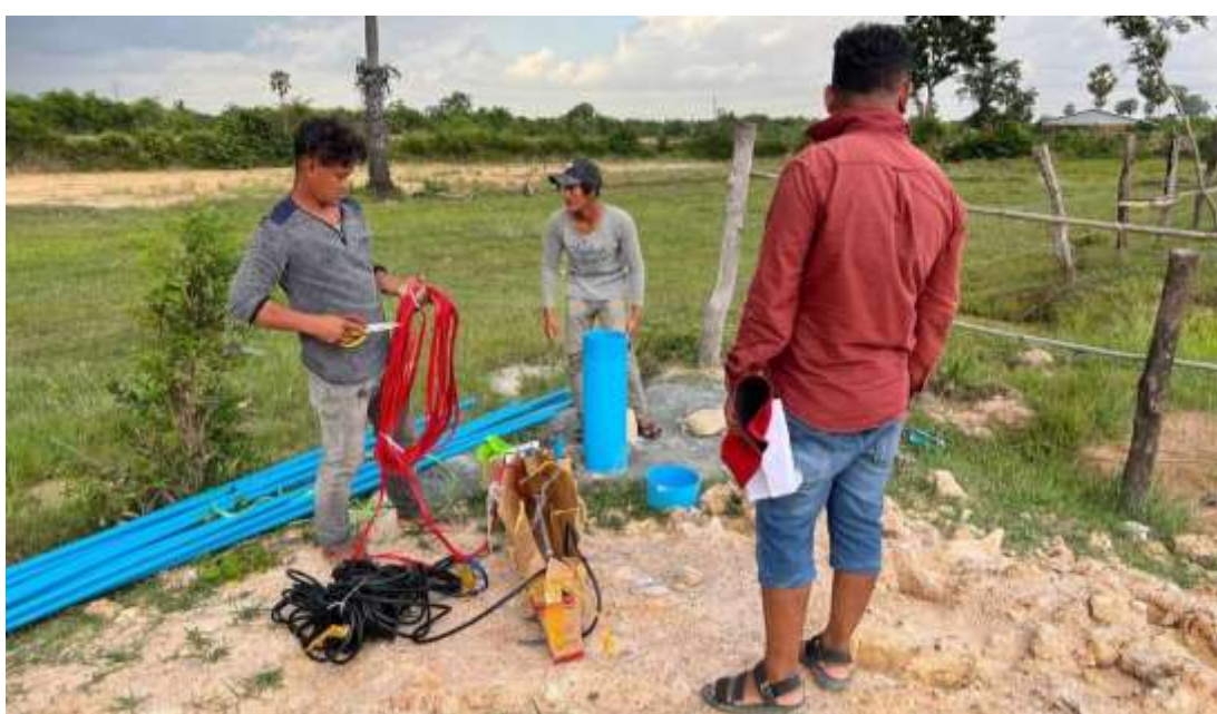
Photo 62: Pumping installation in the borehole at Sek Kong Water Supply and Peng Hong Water Supply
