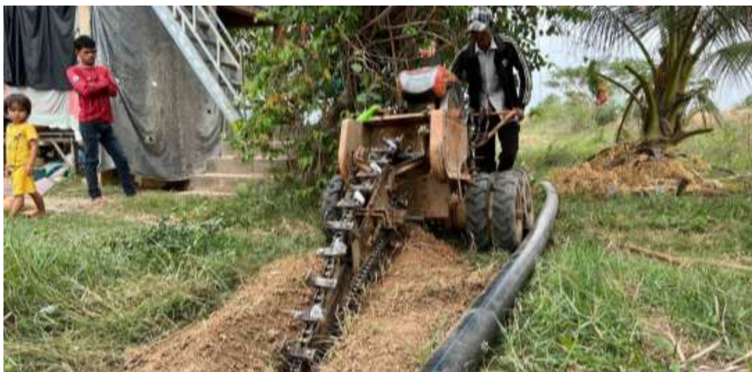
Photo 60: Activity of pipe water supply installation at Krang Chek Water Supply, Kampong Speu province
