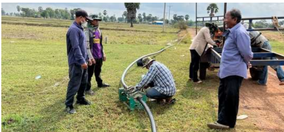
Photo 61: Activity of pipe water supply welding at Veal Pong Water Supply, Kampong Speu province
